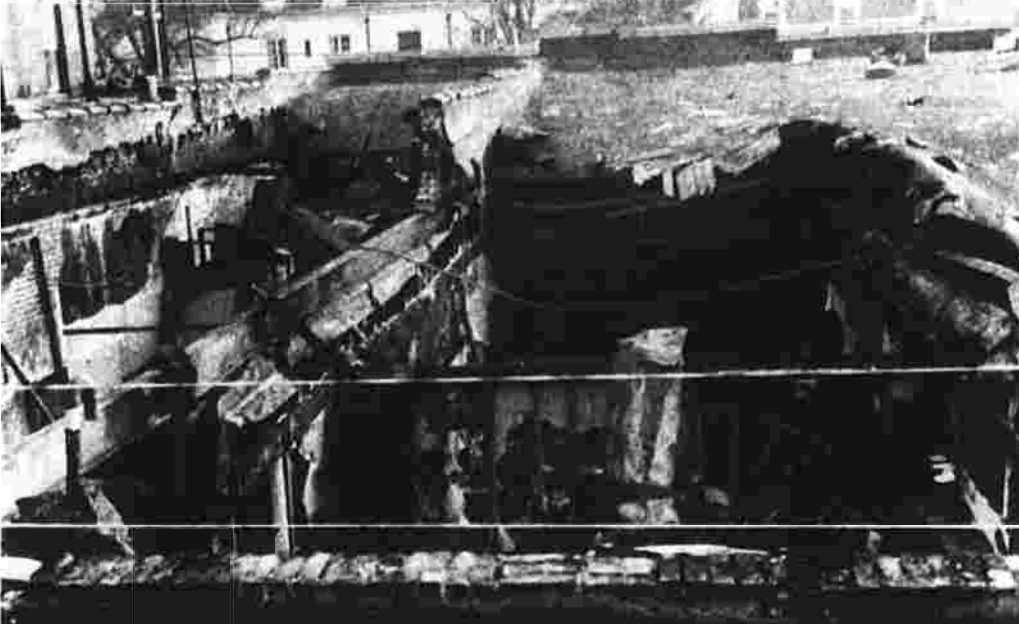
The roof to the rear of the Prichard block on Union Street in Rockville, caved in along the rear of the block, the result of a fire early Sunday. Shown is the storage area of the Star Hardware Store, one of the eight commercial tenants of the building. (Herald photo by Richmond)
