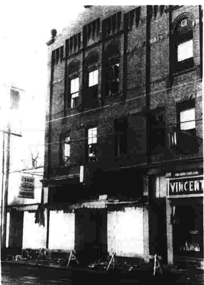
Shredded awnings, broken apartment windows and boarded up store fronts, tell the story of the fire that extensively damaged the 91-year-old Prichard block on Union Street, Rockville, early Sunday morning. (Herald photo by Richmond)
